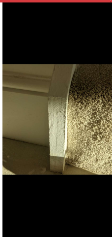
ISSUE 93 Location Staircase Poor workmanship
