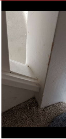
ISSUE 91 Location Staircase Poor workmanship
